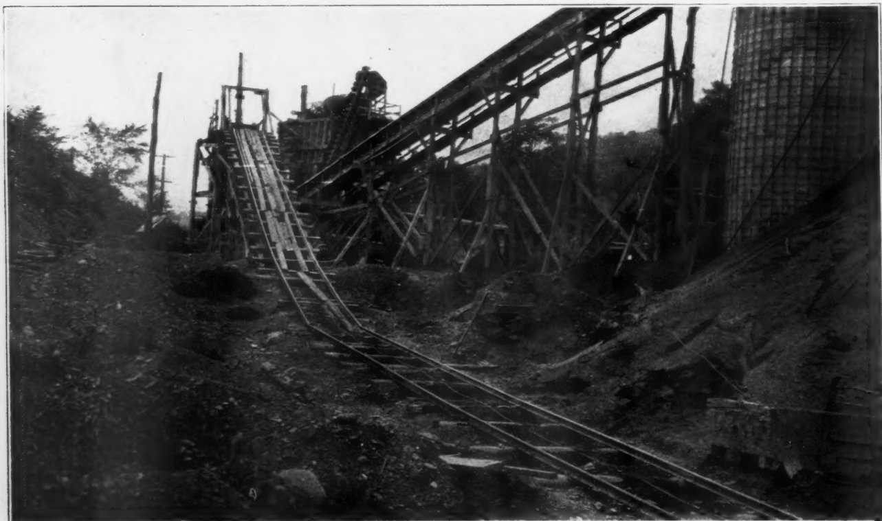
Incline from Quarry to Scalping Screen and Crusher
